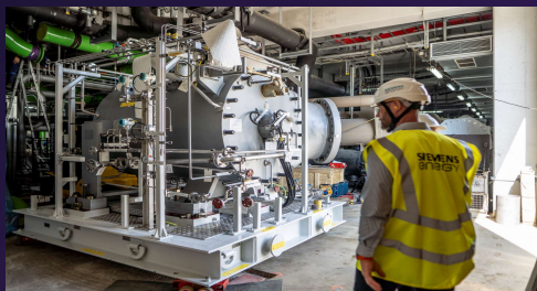
District heating system, Berlin, Vattenfall, Germany
