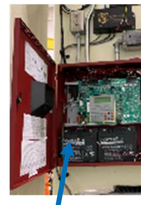
Panel control antincendios
